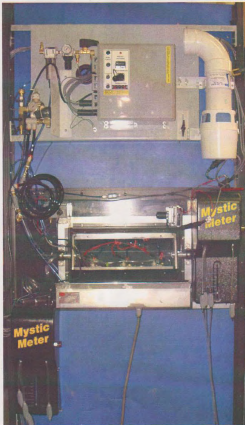
Completed Installation View
